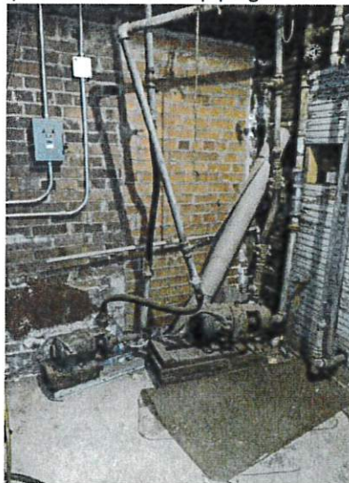
Basement Level Abandoned Pumps and Associated Piping
