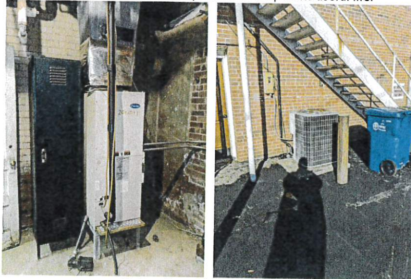
Air Handler #3 / Condensing Unit #3
