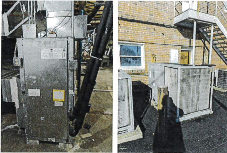
Air Handler #1 / Condensing Unit #1
