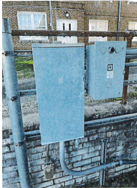
Street Lighting Panel at Rear of Building
