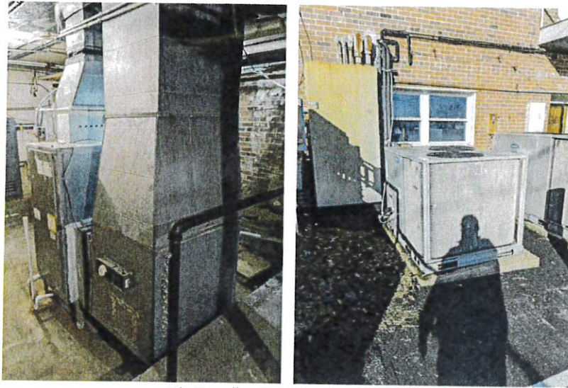
Air Handler #2 / Condensing Unit #2
