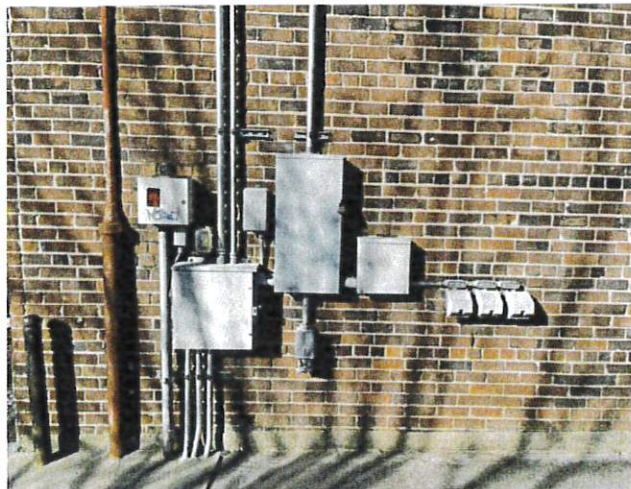
Street Lighting/Shore Panel at Front of Building
