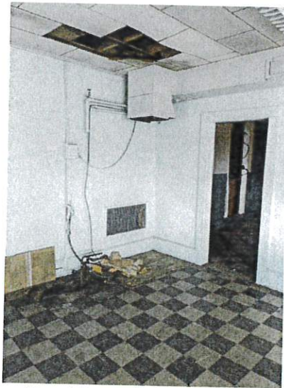
Second Level Exposed Abandoned Ductwork
