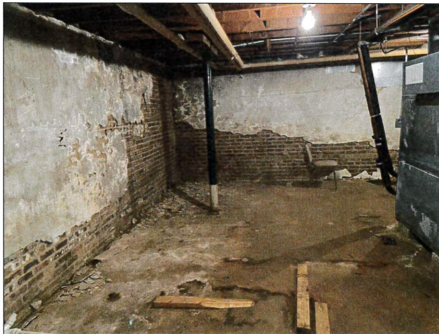
12 - View of plaster delamination in the basement.
