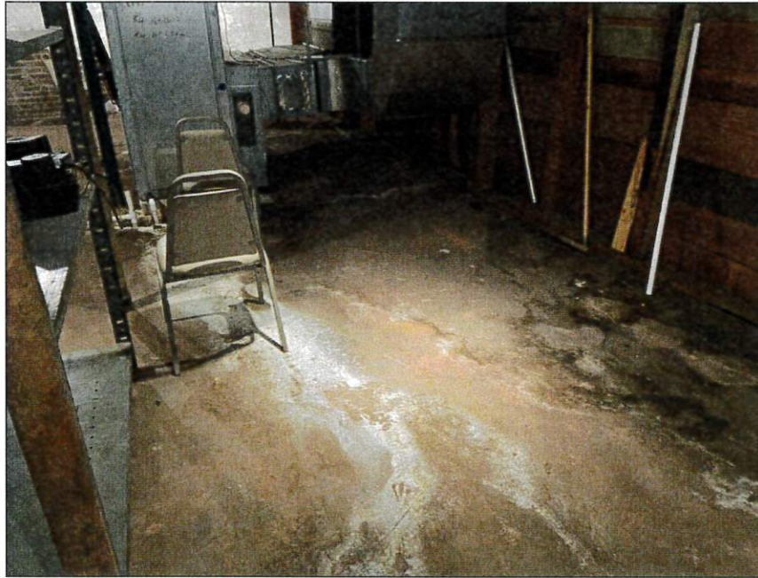
13 - View of water staining on concrete in the basement.
