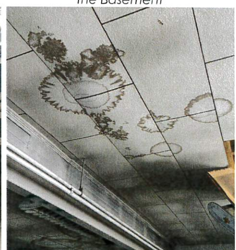
View of Old Roof Leak
