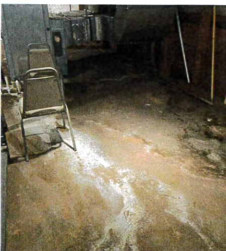
View of Water Staining on Concrete in the Basement
