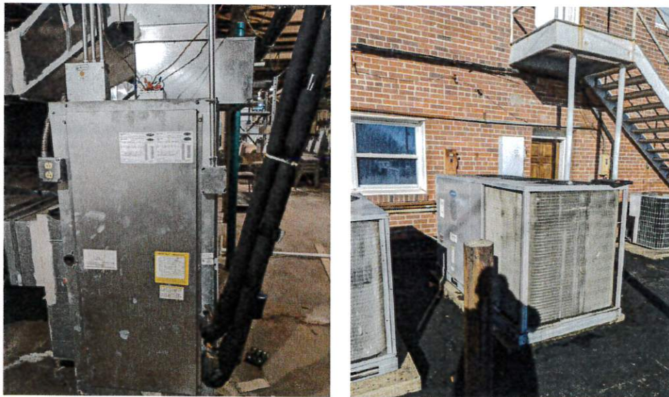
Air Handler #1 / Condensing Unit #1
