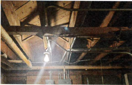
Basement girder that needs a column
