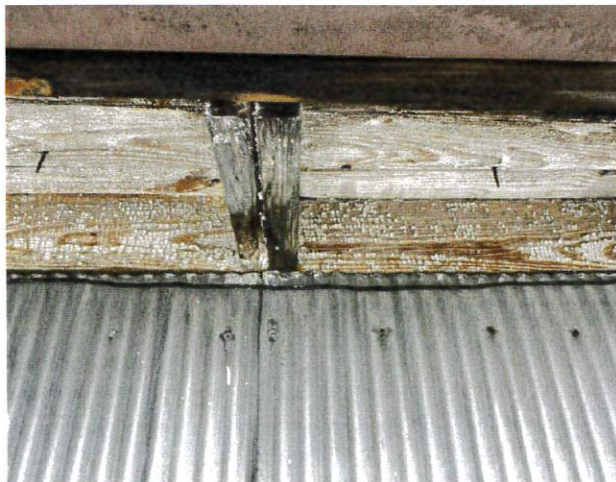
View of White Lead Based Paint
