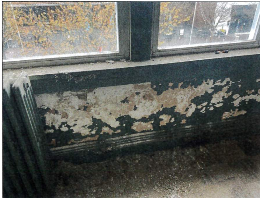
14 - View of plaster delamination below windows
