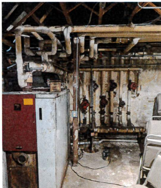
Basement Level Abandoned Boiler and Associated Piping
