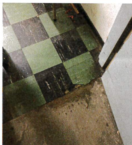
View of Asbestos-Containing Floor Tile
