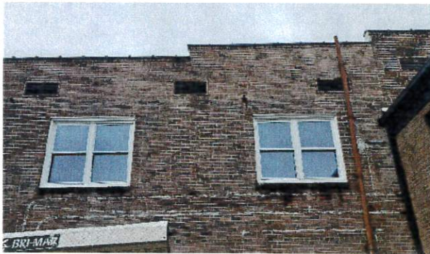
Flashing under windows need addressing
