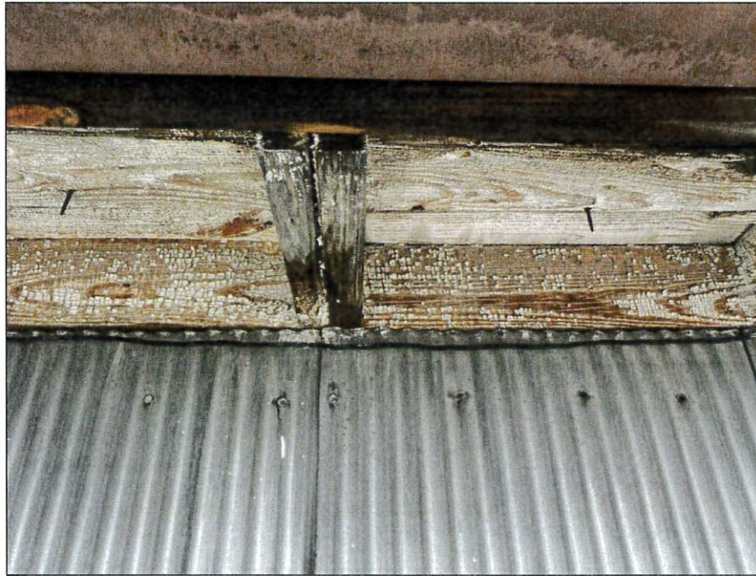
5 - View of white lead based paint
