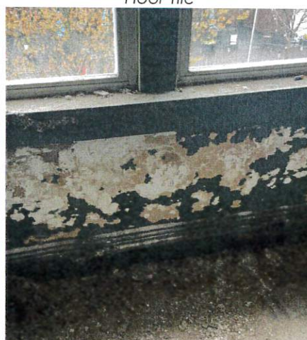
View of Plaster Delamination below Windows
