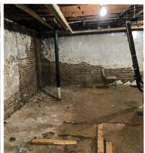
View of Plaster Delamination in the Basement
