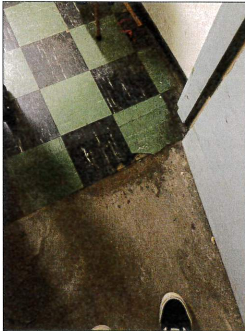
11 - View of asbestos-containing black and green floor tile
