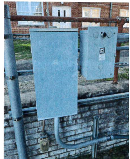
Street Lighting Panel at Rear of Building
