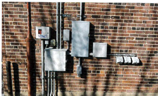
Street Lighting/Shore Panel at Front of Building
