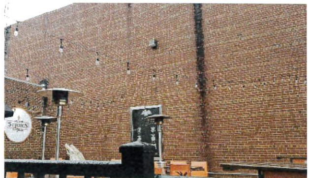
Roof drain from roof in need of repair
