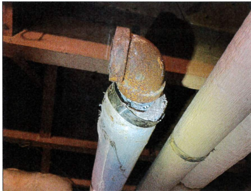
6 - View of air-o-cell pipe insulation
