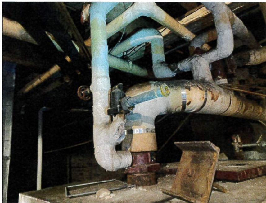
2 - View of asbestos-containing pipe elbows
