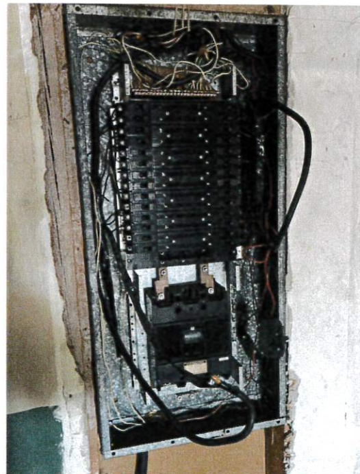
2nd Floor Panel
