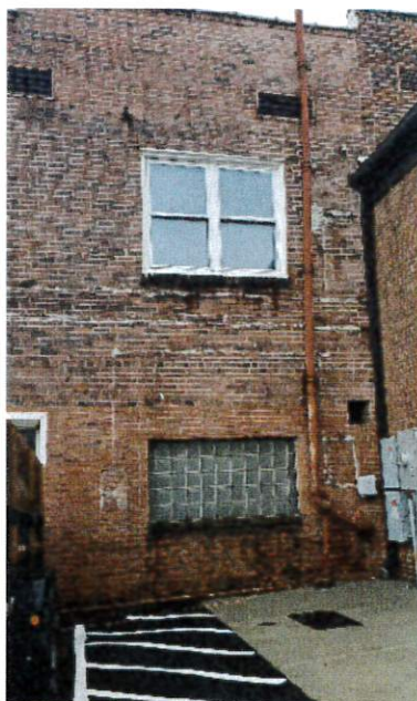
Flashing under windows need addressing
