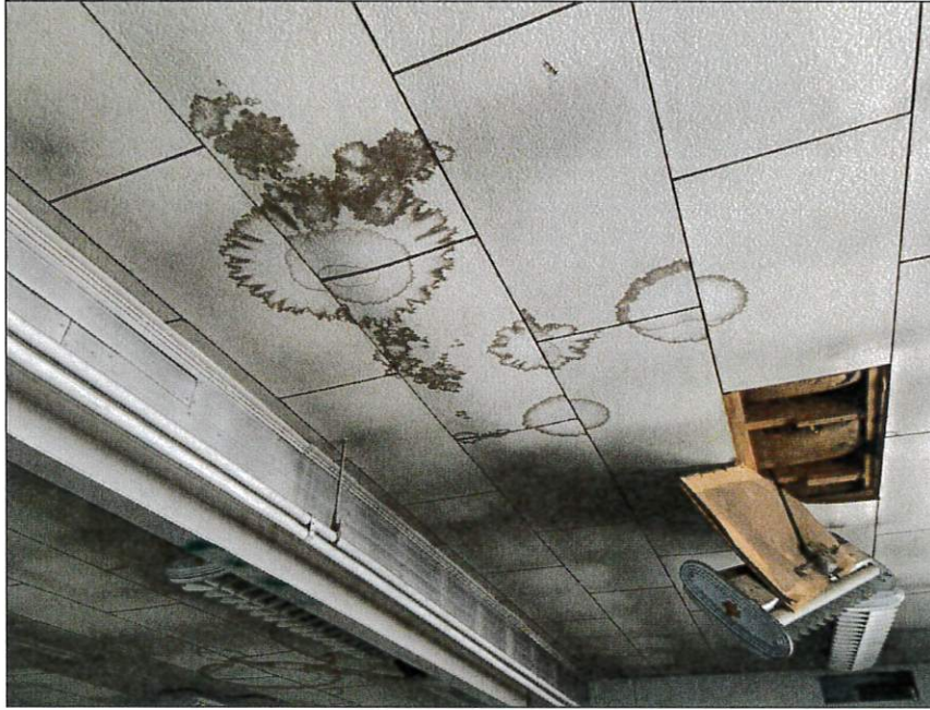
15 - View of old roof leak.
