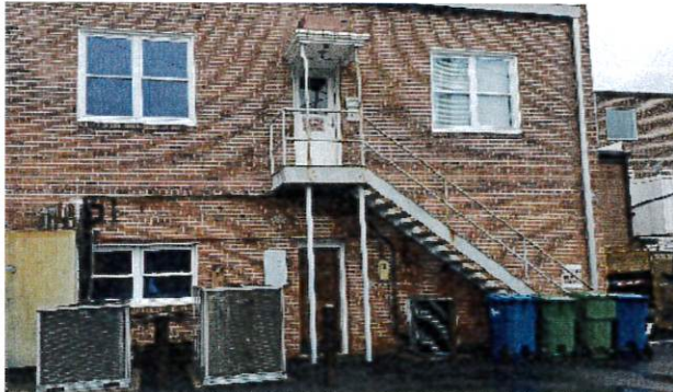
Exterior Stairs that need repair/replace
