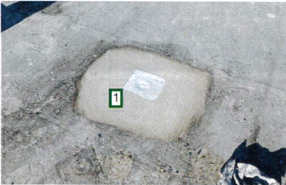
Existing: Upper Roof Existing Core (Location 1) with temporary patch.
